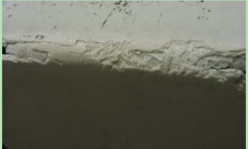
Impossible to clean surface due to de-lamination
